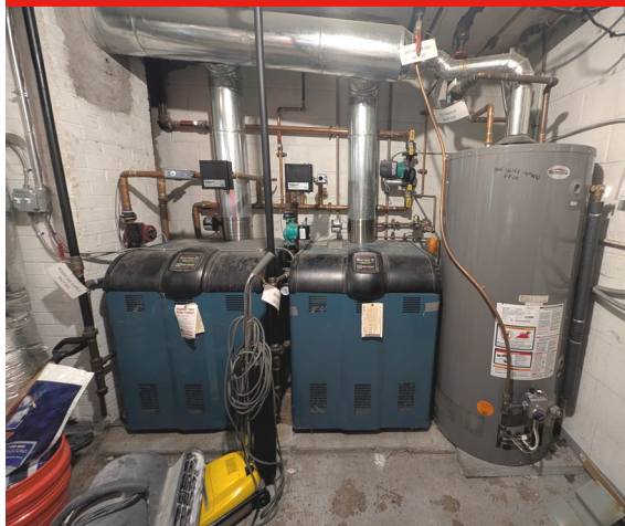
BOILERS / WATER HEATER
